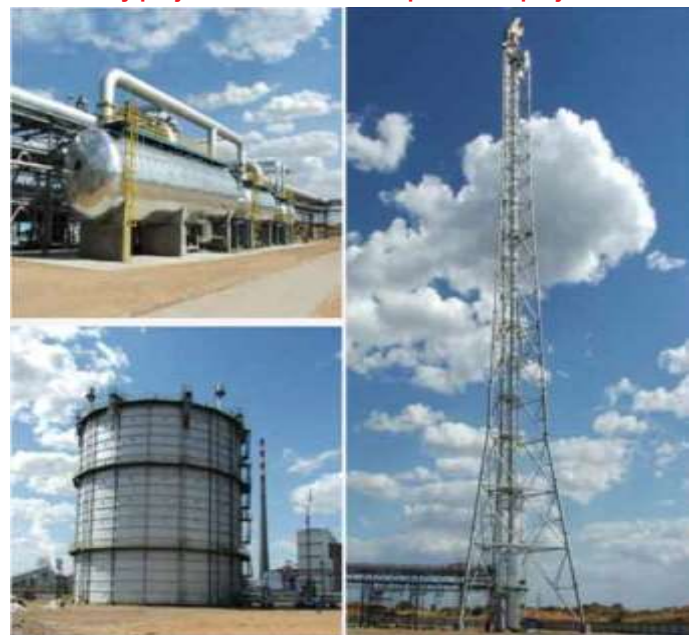
Figure 3: The flare gas & glare gas recovery system used in a national key project “Shenhua coal liquefaction project”.
